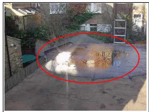
Leaks can be caused by ponding on a flat roof
