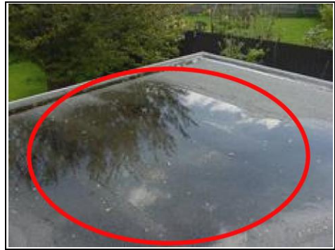
Ponding on a flat roof
