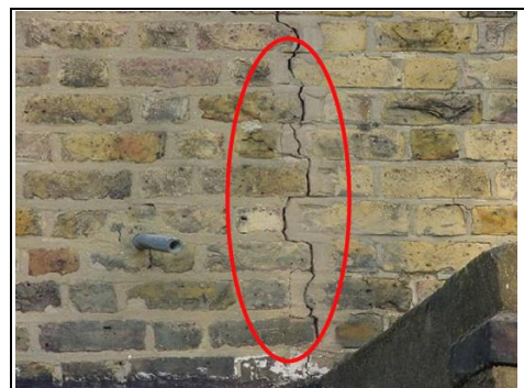
Movement causing cracks in the brickwork
