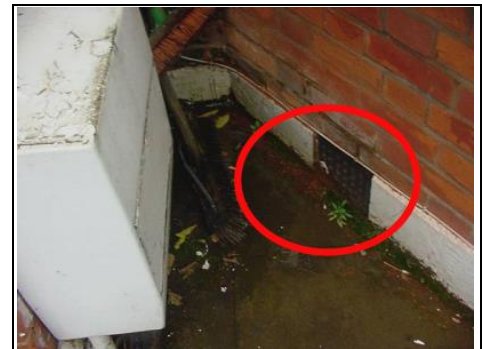
Air brick acting as gutter causing dampness internally
